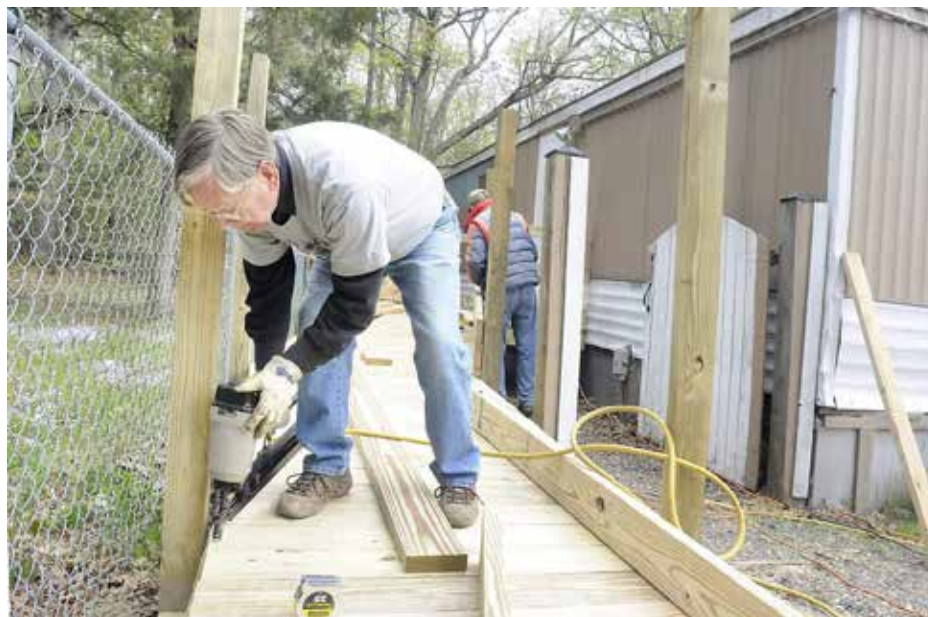
(Photo by GREG DOHLER) Kiwanis Club of Waldorf member Ernie Wallace of La Plata helps build a wheelchair ramp at the home of Calvin Cooper as part of Christmas in April on Saturday in Welcome.
